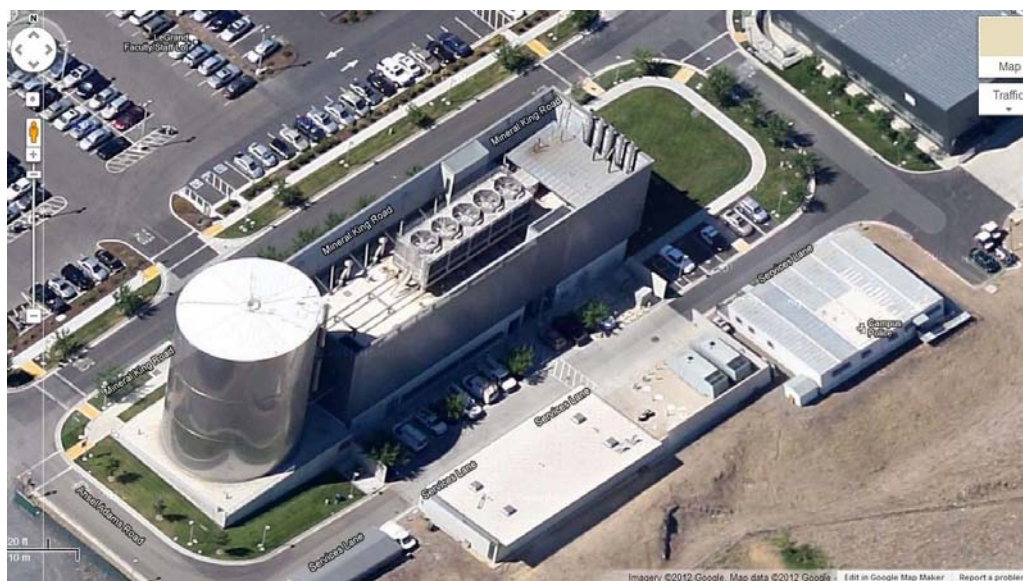
Chilled Water Storage
